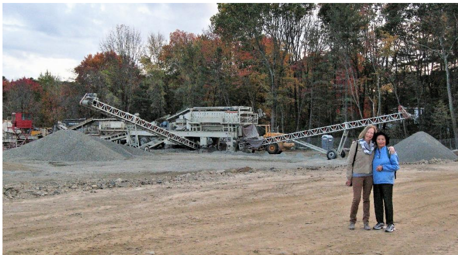
Neighbors tour the construction site on 10/23/2017. Residents were unaware that placement of the large rock crusher near Mill Street residences violated the Construction Mitigation Plan.
